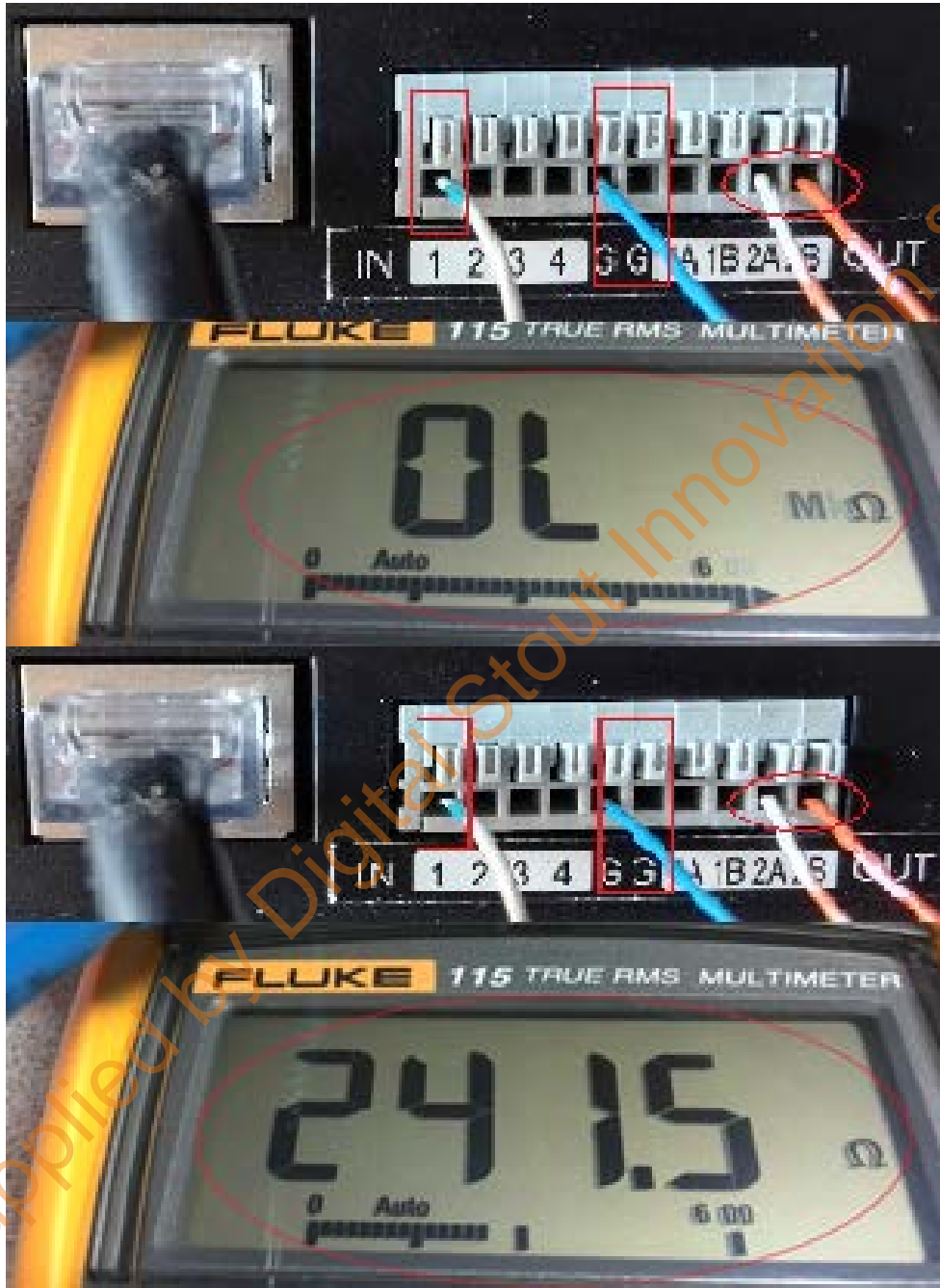
Figure 25-4: GVR355X Alarm_Out Circuit Measurement
